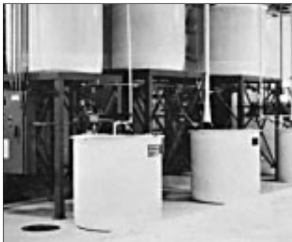
Industrial waste water treatment facility.
